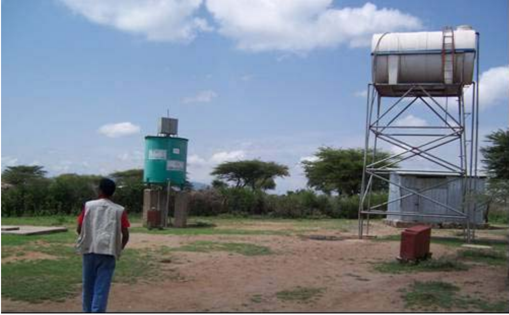
Defluoridation plant at Langanu PA.
